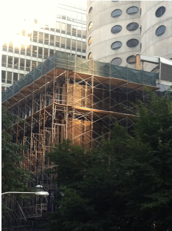
Scaffolding was placed at Prentice’s Miesian base as demolition began in mid-2013.
